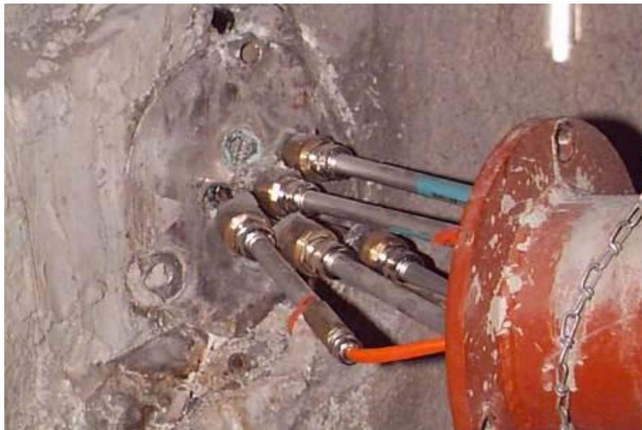
Figure 5.7: Damaged displacement transducers of the extensometer
