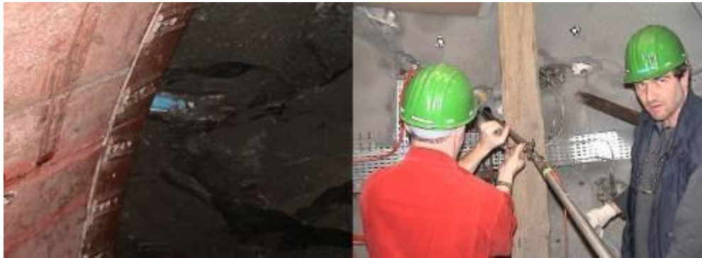
Figure 8.15: Inclinator B1 : casing as seen from the tunnelling shield (left); the chain is partly recovered from the Test Drift side (right)
